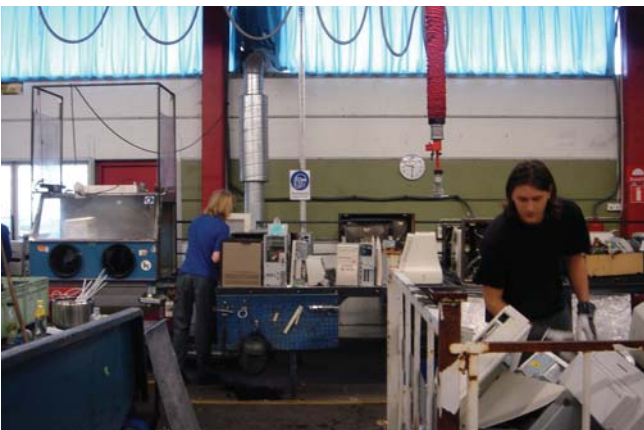
Exhibit 5.4 Cabinet for removal of hazardous dust
